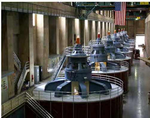
The generators inside the hydroelectric power plant.
